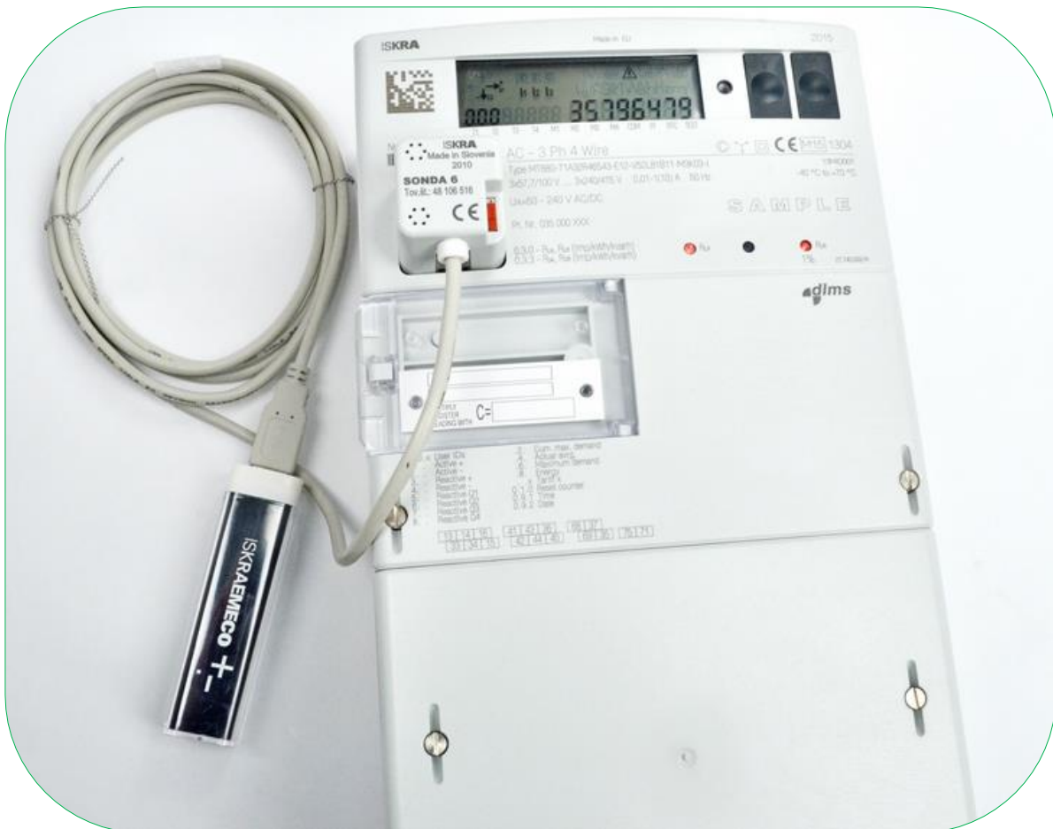
Figure 92: No power reading – meter supplied by power bank via optical probe
